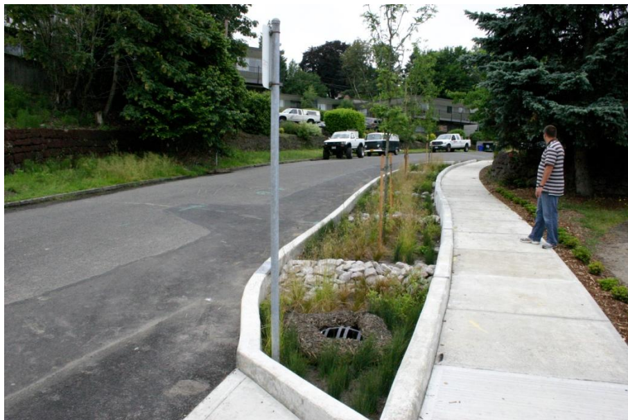
Mid-block curb extension with bioswale (Credit: Brad Lancaster)
