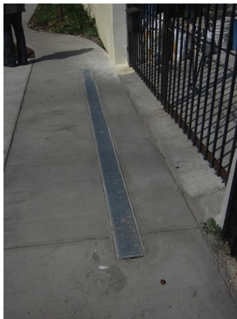
Trench drain in hardscape (Credit: Stephanie Landregan)
